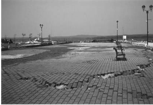
Photo 7 Crack of stone pavements and traces of sand blow phenomenon (left).
