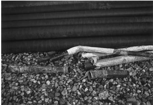
Photo 8 Broken pipe of thermal water caused by the 2007 Earthquake.
